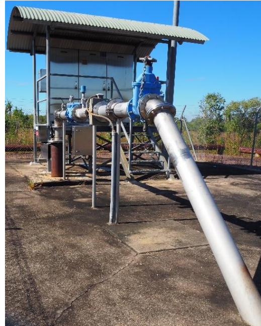
Photo 4: Pump at Howard East borefield, May 2021
