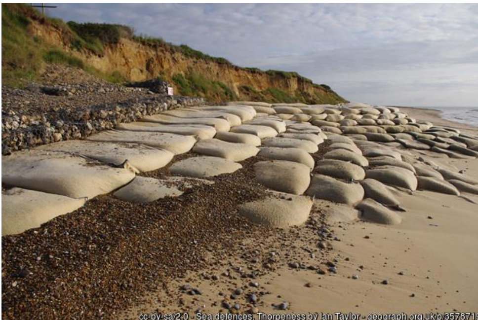
Large sandbags used to prevent erosion (Image credit at bottom of photo)
