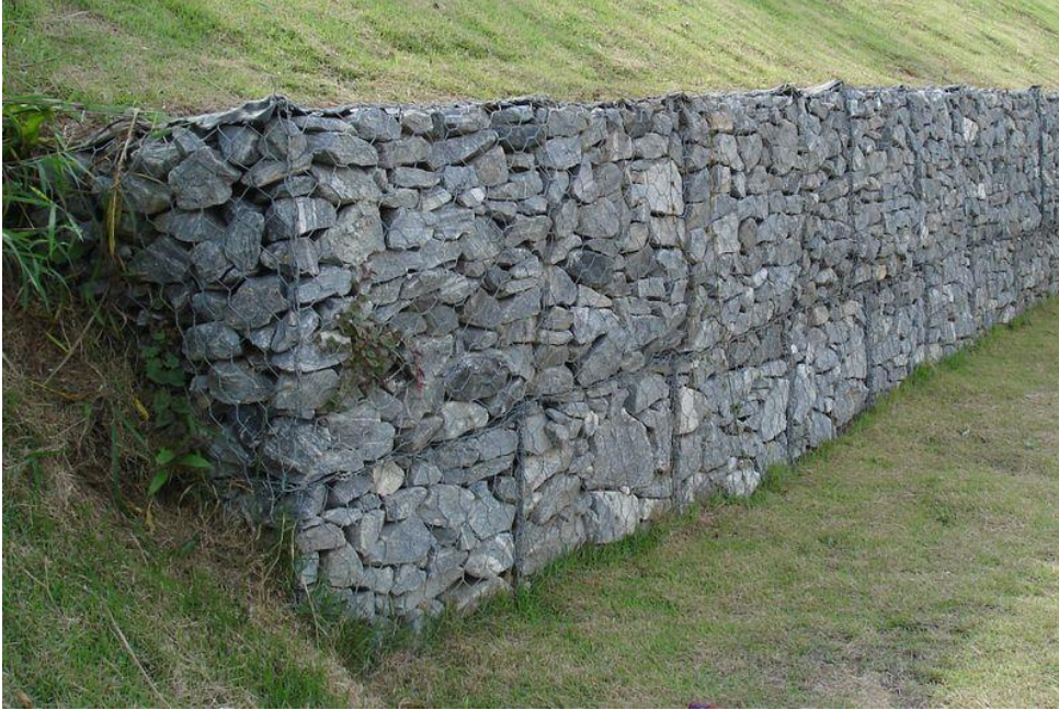
Gabion (rocks held in wire cages) used to prevent erosion (Image: Wikipedia Commons)
