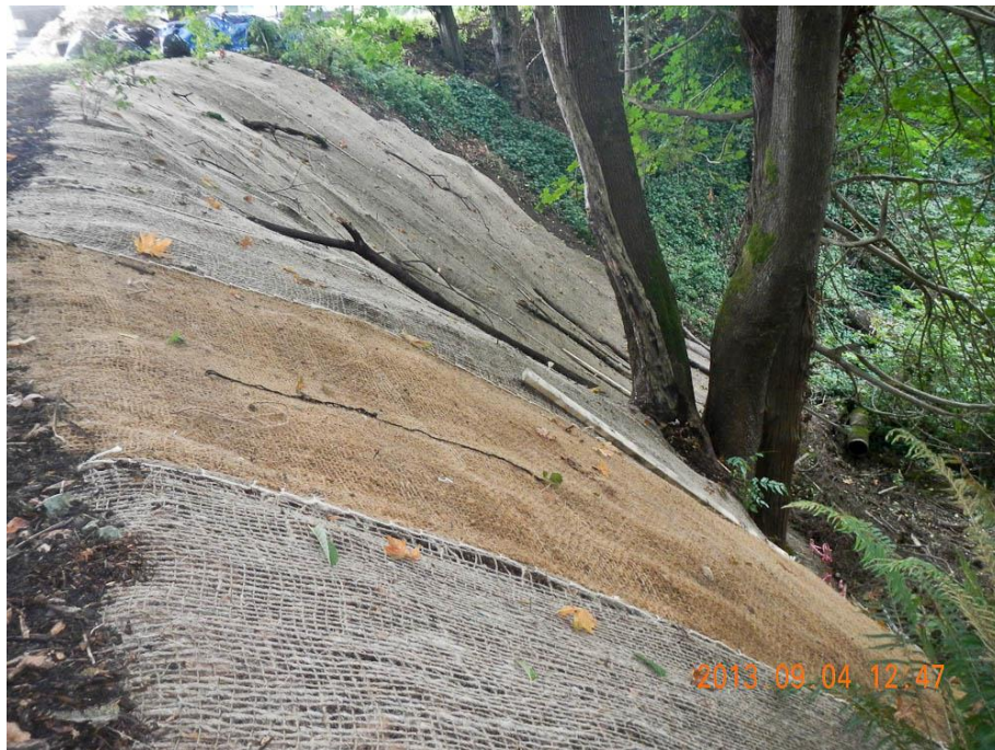
Jute netting on a slope to prevent erosion (Image: Luke McGuff via flickr.com )
